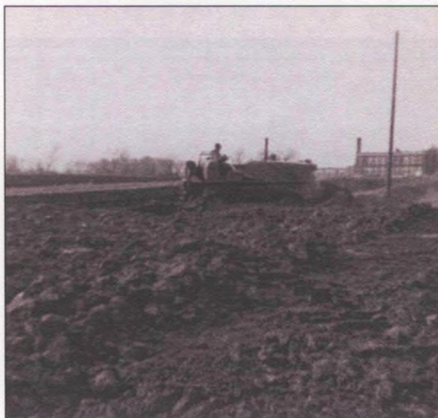
Construction of Minnesota Highway 83 mid 1950s (note the school in the background)
